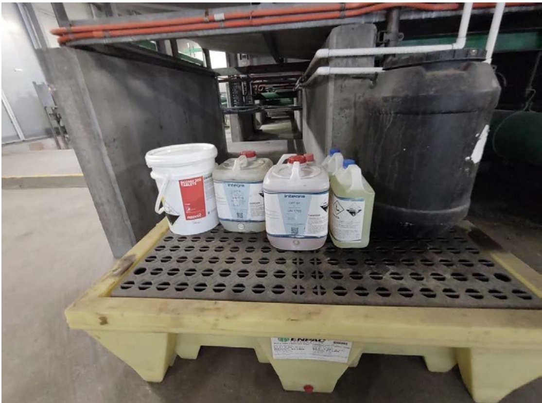
Photo 6: Chemical containers stored in cooling tower room
