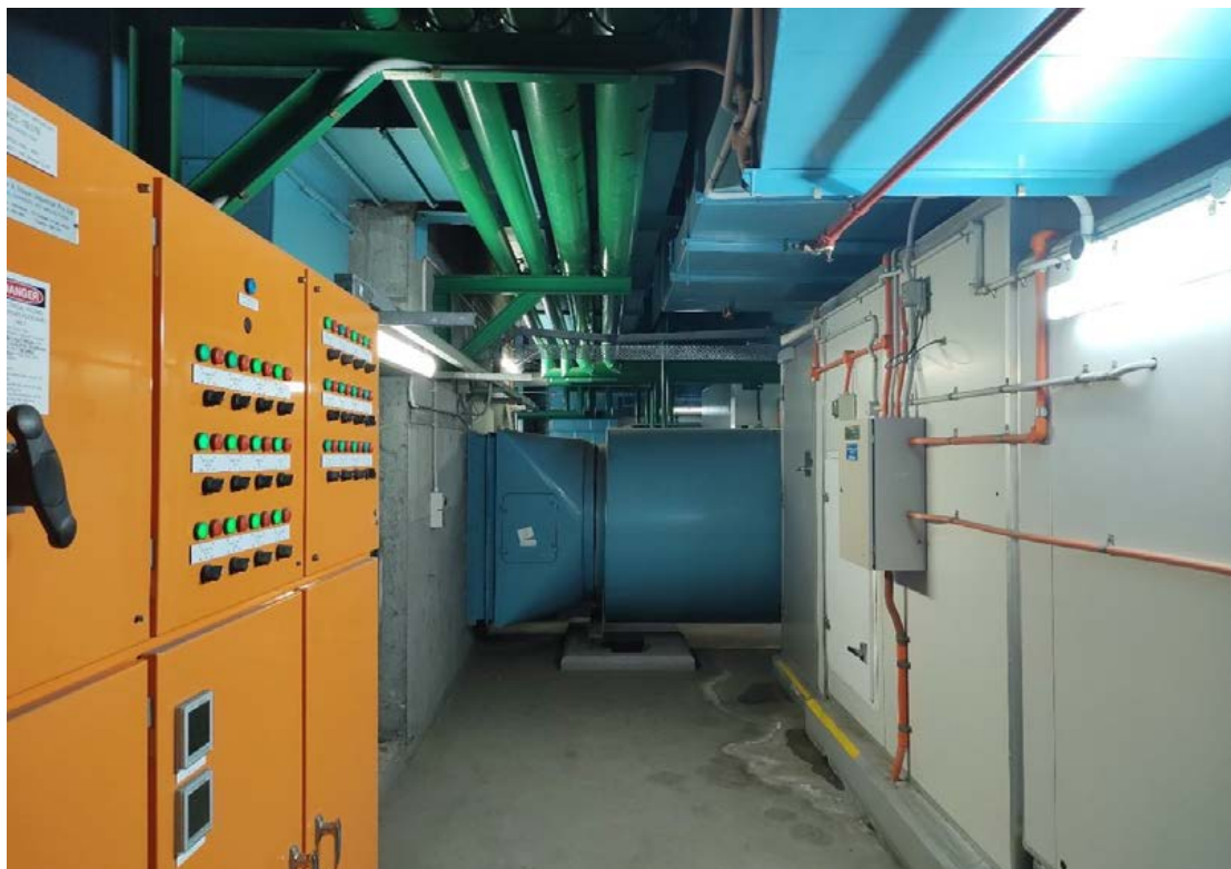
Photo 1: Plant room in level 19
