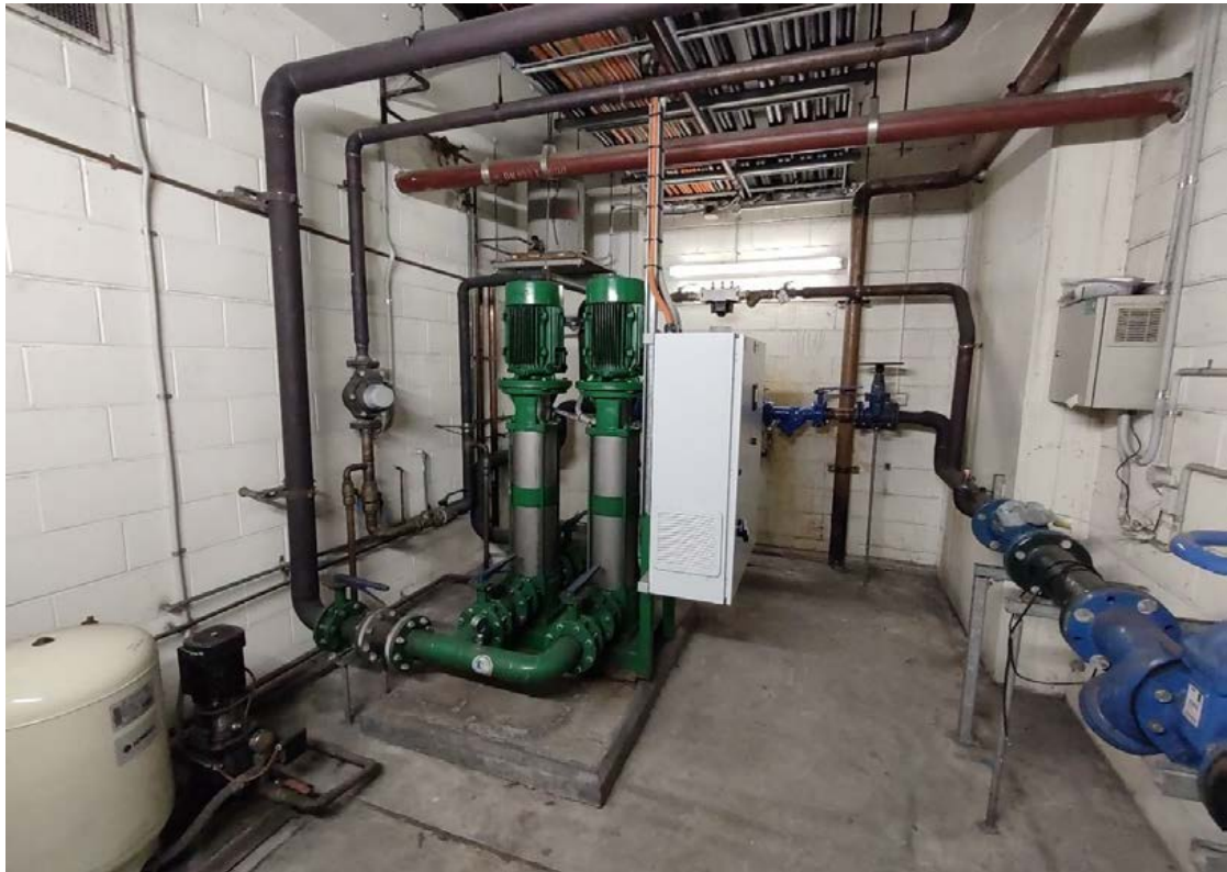
Photo 19: Water pump room in basement 2
