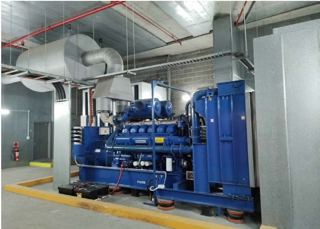
Photo 11: Diesel generator room in level 7
