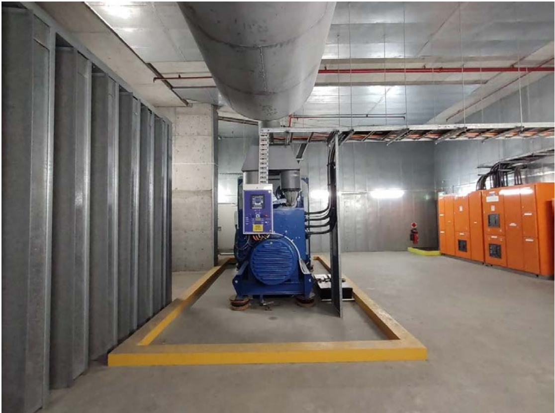
Photo 12: Diesel generator room in level 7
