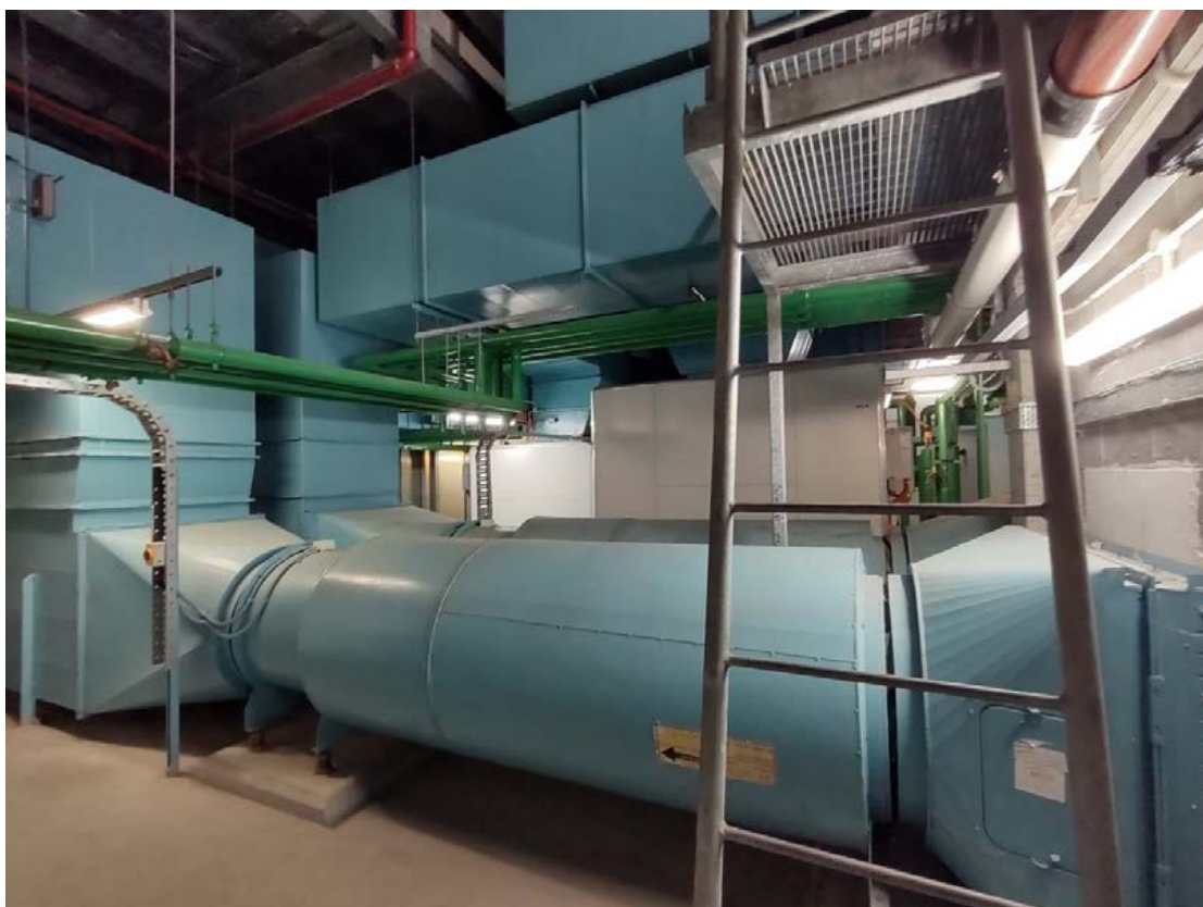
Photo 2: Plant room in level 7
